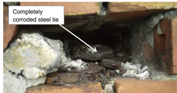
Fig. 2. Total corrosion of the steel tie.
