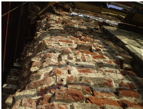
Fig. 8. Destruction of the solid bricks visible on the surface of the load-bearing layer.
