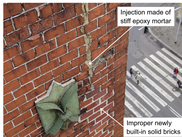
Fig. 9. Improperly made repair works, which are escalating the further destruction.
