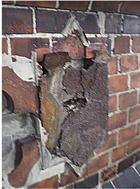
Fig. 3. Remains of the corroded steel anchor plate
